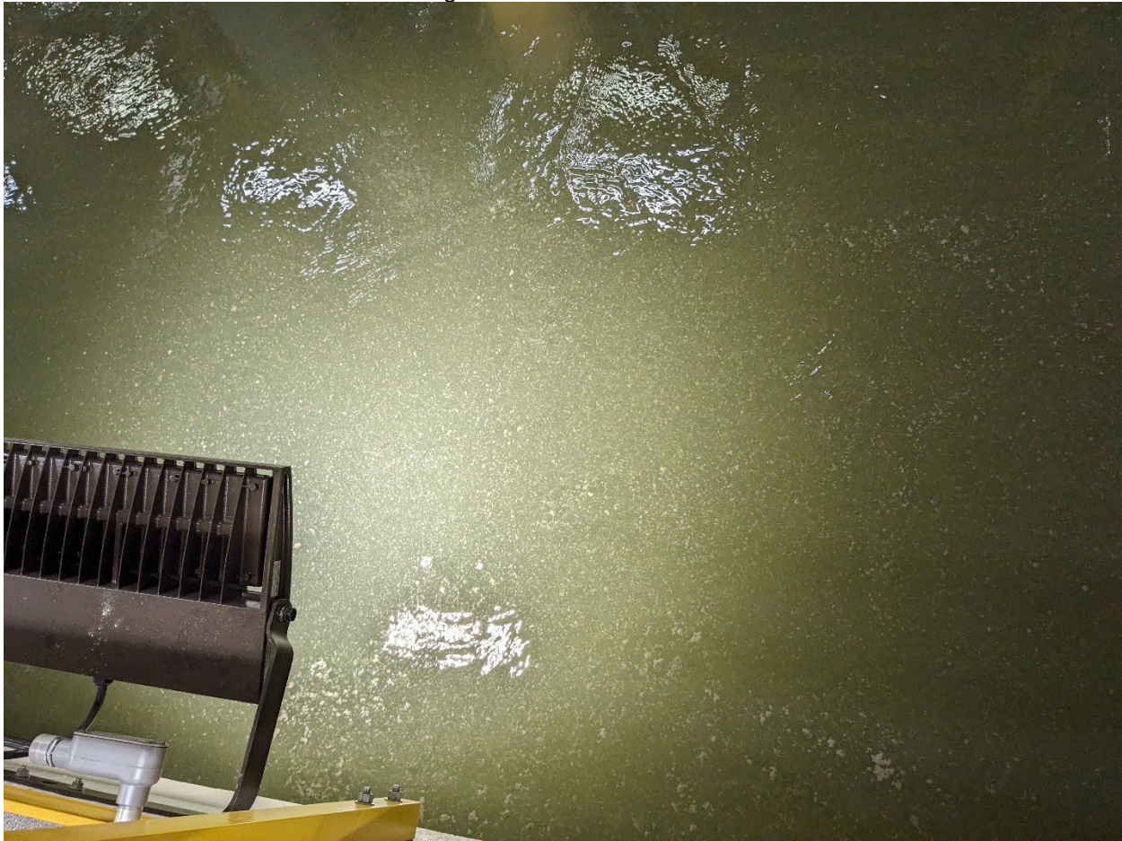
Pin Flocculation in Flocculation tank during Disc Filter Test Runs
