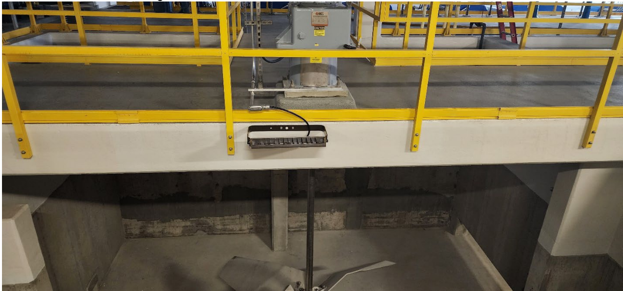
New flocculation basin light installed
