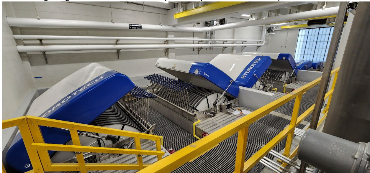
Disc Filters getting the mechanical checkouts, covers open and backwash system extended
