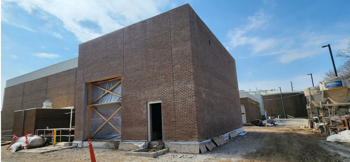
Another view of new Chemical Storage Room, new brick matches very well with existing structure 60
