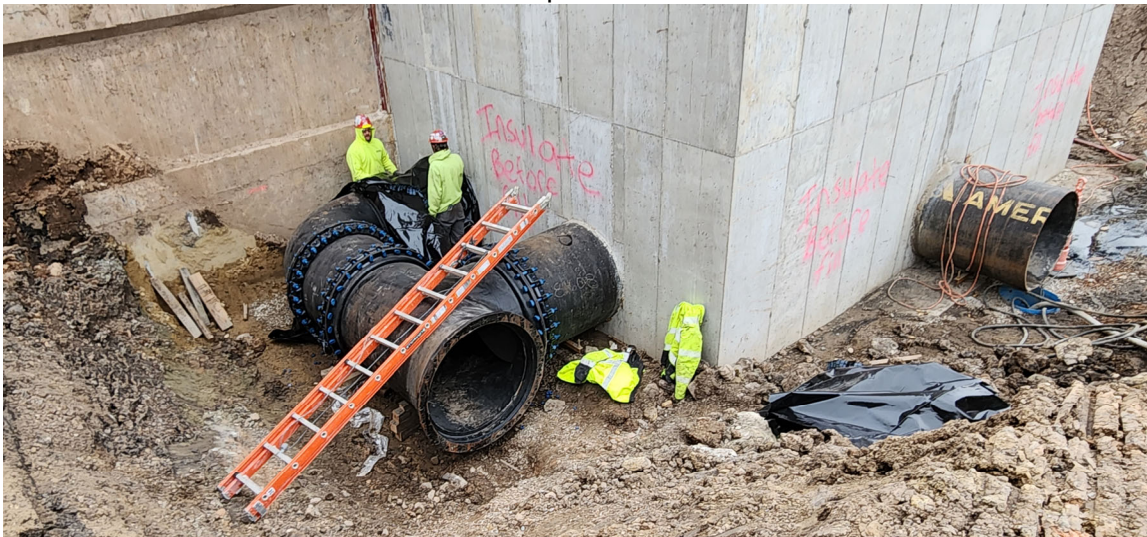
42-in. SE lines extended out of the west wall of Filter Splitter Box
