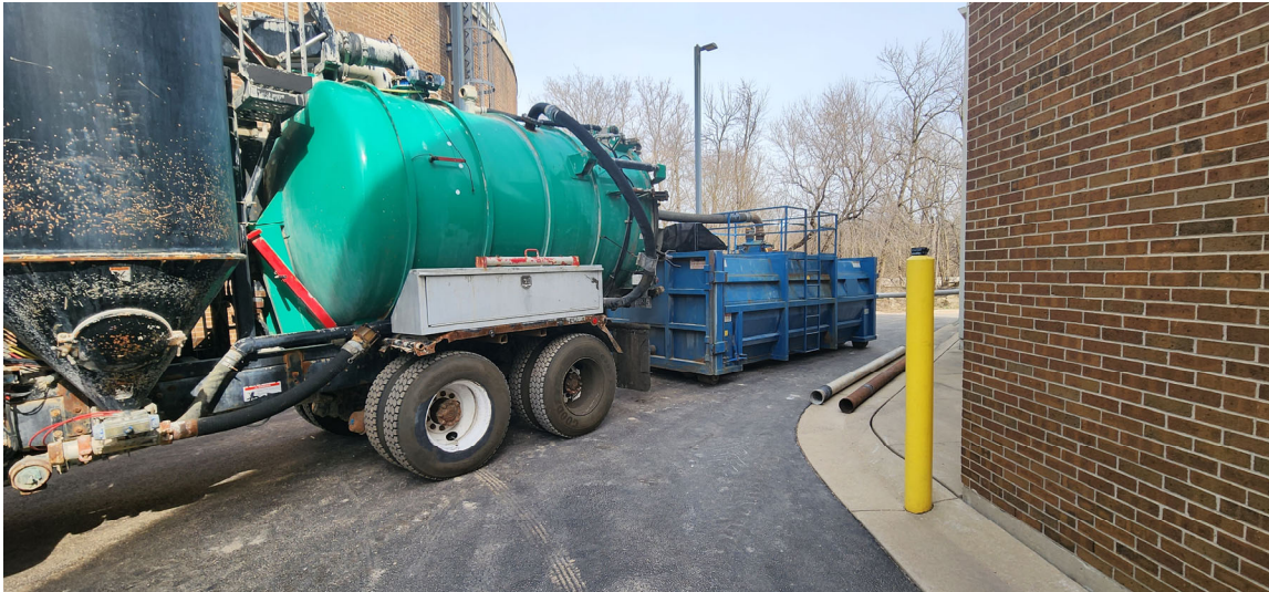
CD Smith preparing for cleanout of Back Wash Tank with Vac Truck to allow for structural inspection of concrete
