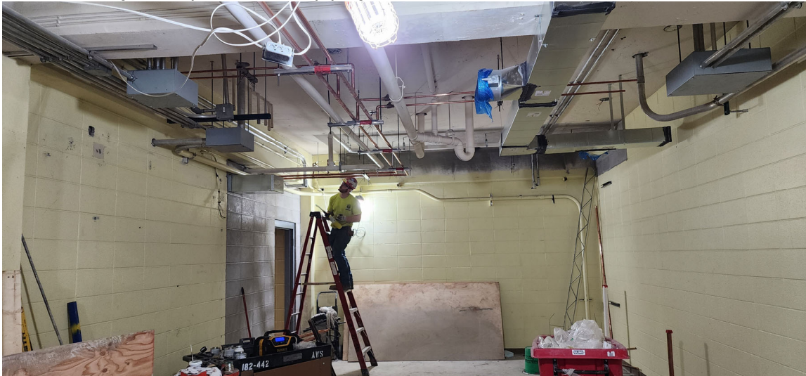
August Winters working on the potable water piping in the Women's Locker Room
