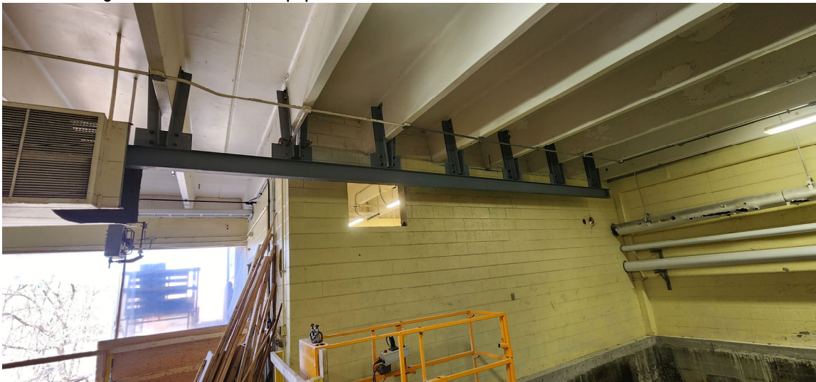
Iron workers installing the first disc filter equipment monorail for disc filter #1
