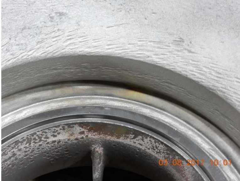
Suction Bell: Wear ring fit and suction bell erosion from pumped media.
