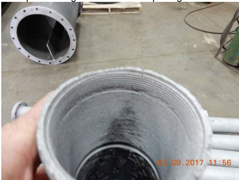
Top Enclosing Tube: Top threads show severe washout and wear.
