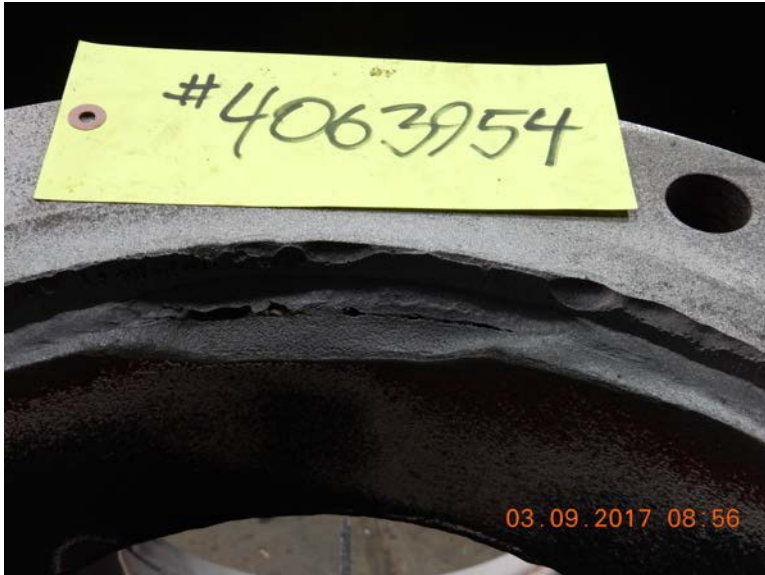
Discharge Head: Discharge flange fit shows evidence of wash out and requires repair.
