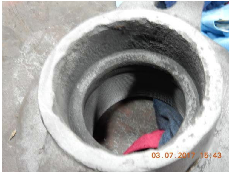
Packing Box: The packing box bore is oversized and severely pitted.
